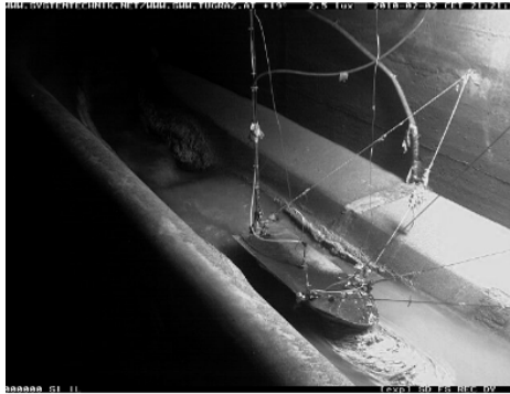
Figure 10.3 View of the overflow chamber and floating pontoon (remote shot from the installed camera, 2010 02 02).
