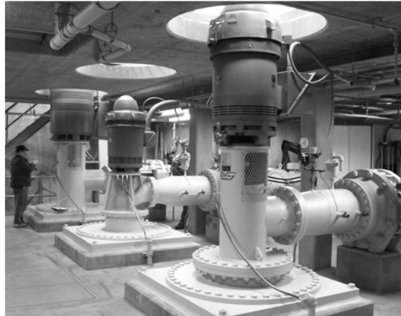
Figure 14.2 Vertical turbine pumps.
