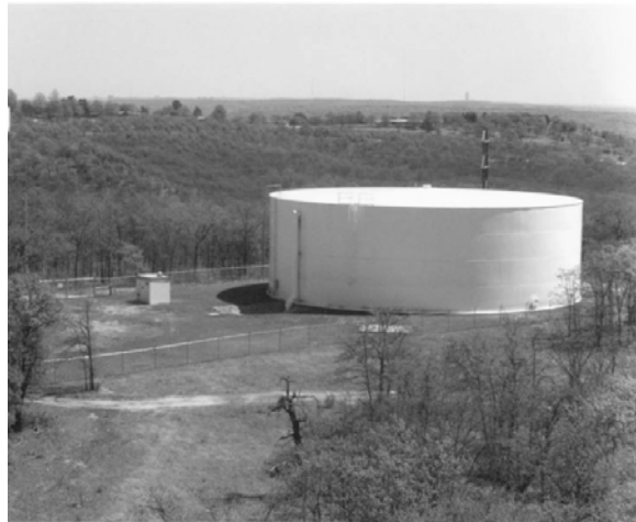
Figure 14.4 2-MG storage tank.
