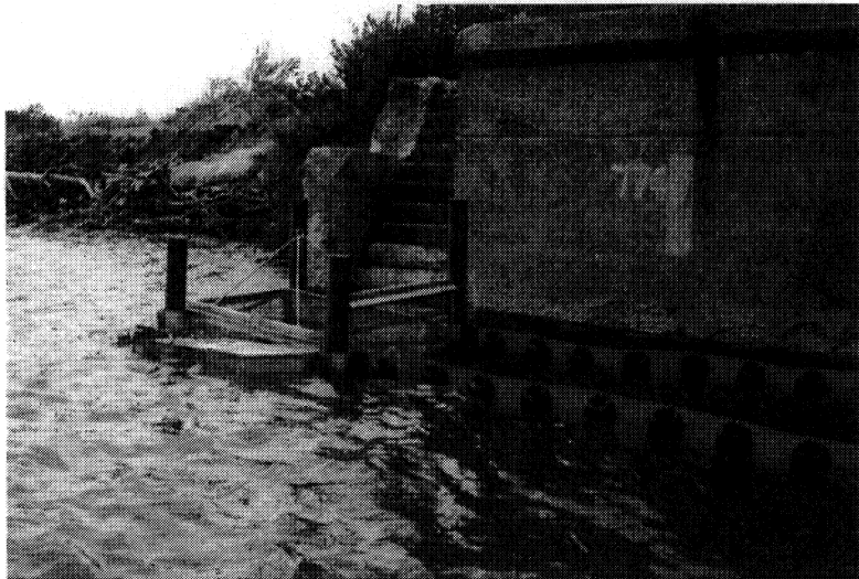
Figure 10.2 (top) Floatables trap at the mouth of the Babcock St. combined sewer outfall. The tide water slide system is visible on the piling in the foreground. This system enabled the boom to rise and fall with changes in water level. A Datasonde was hung from the boom near the piling in the foreground. (bottom) Close up of galvanized steel frame on pontoons (lined with removable nylon net).
