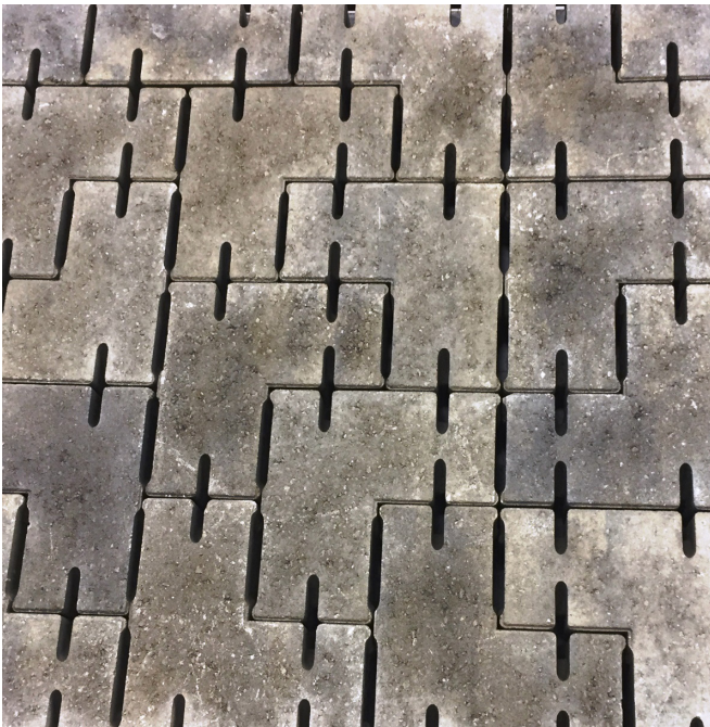
Figure 2 Pavement constructed from two forms of L-shaped PICP blocks with cupules of two different lengths aligned in the direction of sweeper travel; real cupules have rounded edges, cupule width is 12.5 mm, block joints are typically 2 mm wide.
