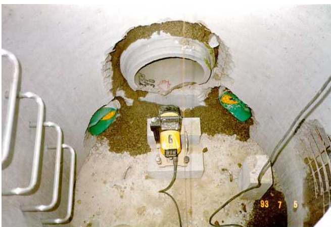
Figure 10 Construction of PVC pipe plugs at both sites of the perforated pipes.
